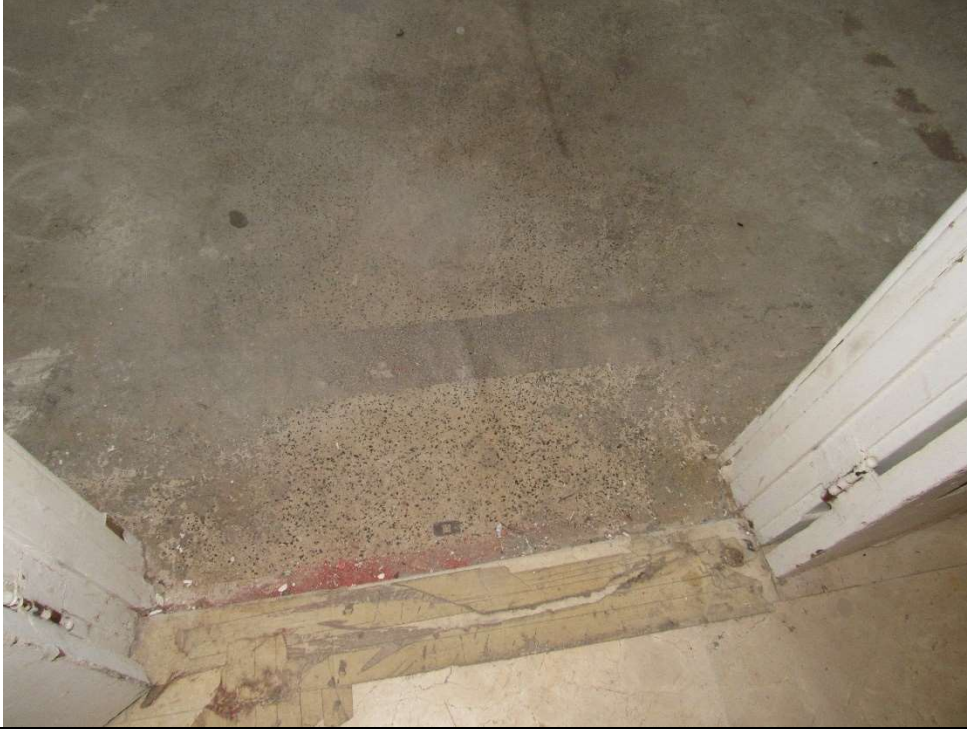
Photo #23 Gulfstream Hotel Building 1 Lake Ave, Lake Worth, FL 33460 Close-up of flooring front room entryway (5/12/2017)
