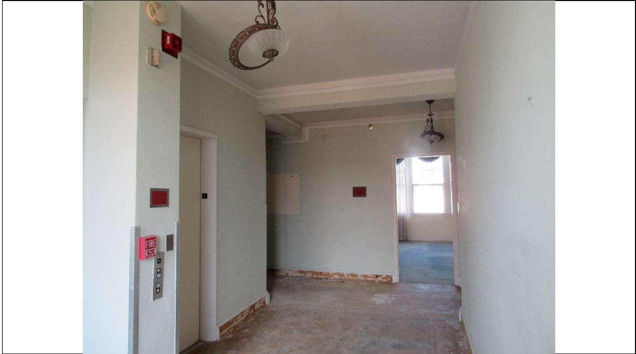
Photo #62 Gulfstream Hotel Building 1 Lake Ave, Lake Worth, FL 33460 Fifth floor elevator lobby (7/10/2020)
