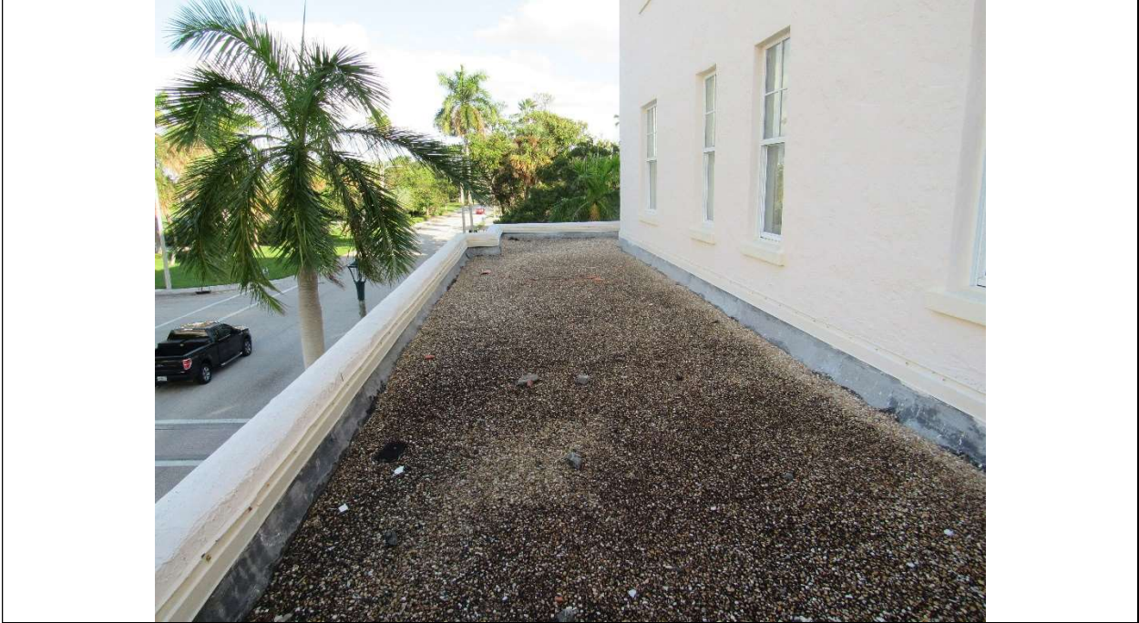
Photo #48 Gulfstream Hotel Building 1 Lake Ave, Lake Worth, FL 33460 Exterior N elevation facing East (5/12/2017)
