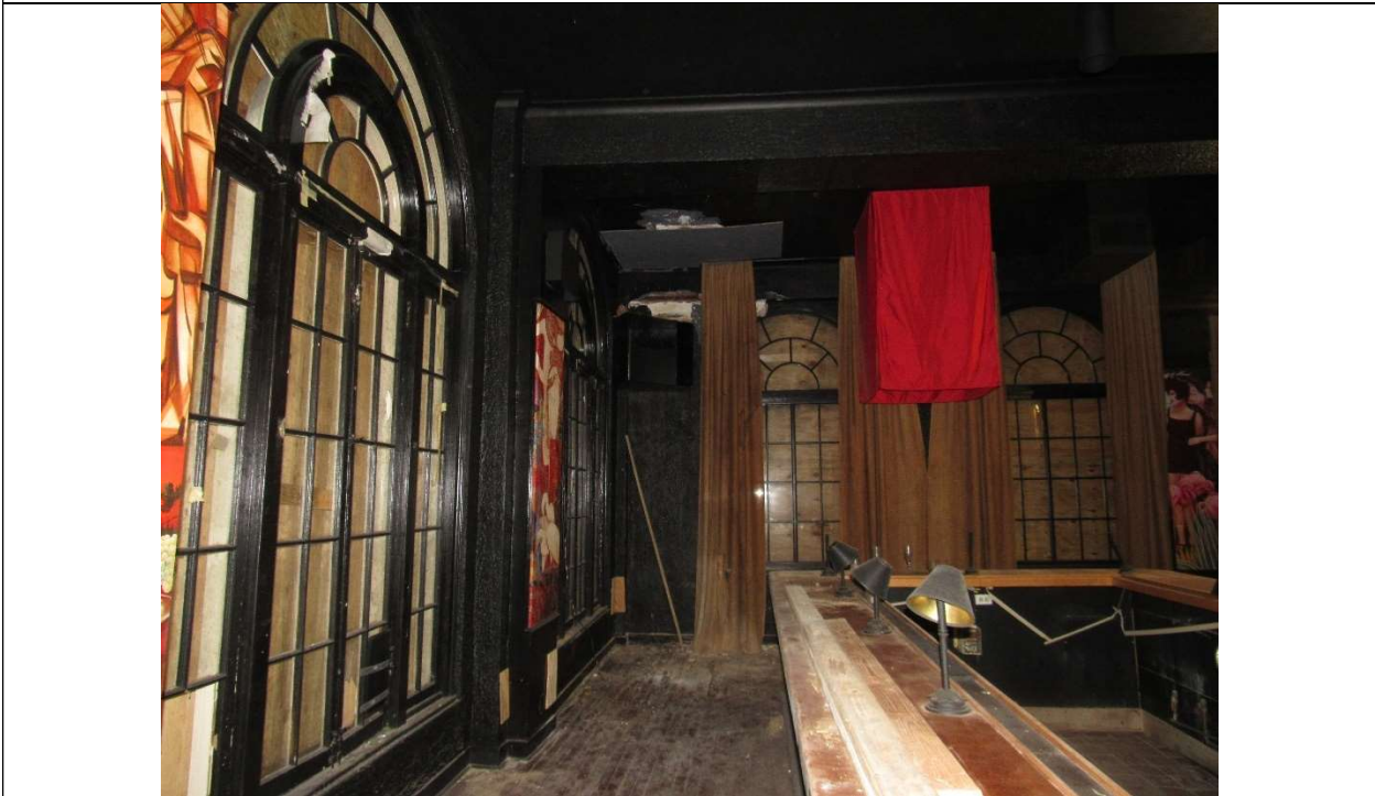
Photo #28 Gulfstream hotel Building 1 Lake Ave, Lake Worth, FL 33460 East wing facing N (7/10/2020)
