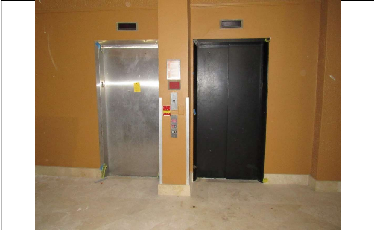
Photo #21 Gulfstream Hotel Building 1 Lake Ave, Lake Worth, FL 33460 Existing elevators in lobby (11/7/2019)
