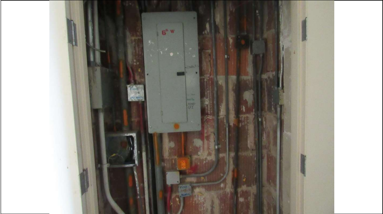
Photo #72 Gulfstream Hotel Building 1 Lake Ave, Lake Worth, FL 33460 Sixth floor electric panel (7/10/2020)
