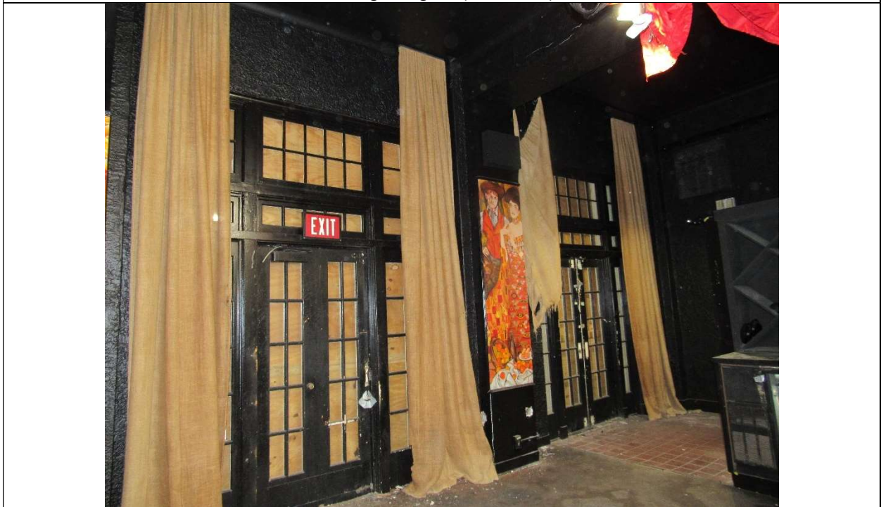
Photo #30 Gulfstream Hotel Building 1 Lake Ave, Lake Worth, FL 33460 East wing facing N elevation doors (boarded from exterior) (11/7/2019)
