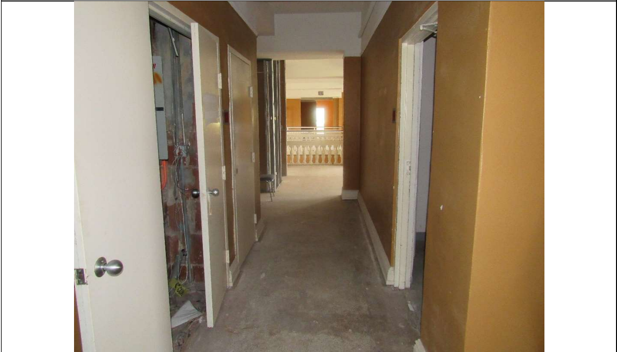
Photo #49 Gulfstream Hotel Building 1 Lake Ave, Lake Worth, FL 33460 2 nd floor corridor (7/10/2020)
