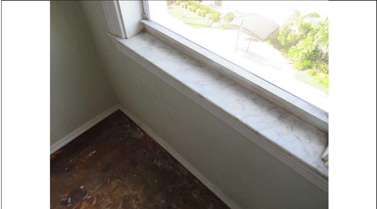
Photo #68 Gulfstream Hotel Building 1 Lake Ave, Lake Worth, FL 33460 Fifth floor window detail (7/10/2020)
