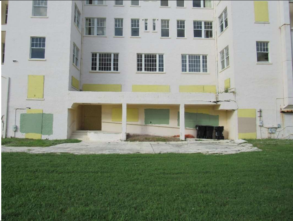
Photo #7 Gulfstream Hotel Building 1 Lake Ave, Lake Worth, FL 33460 Close-up of S Elevation (11/7/2019)
