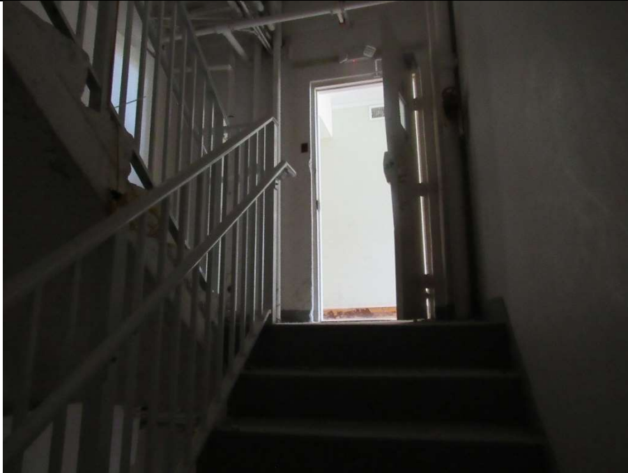
Photo #51 Gulfstream Hotel Building 1 Lake Ave, Lake Worth, FL 33460 Stairwell to third floor (7/10/2020)
