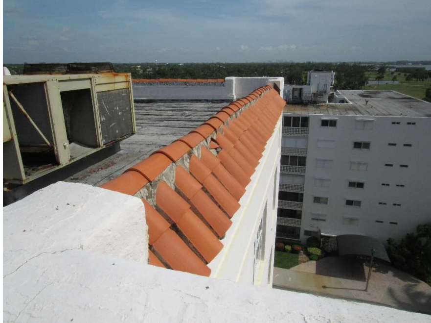
Photo #78 Gulfstream Hotel Building 1 Lake Ave, Lake Worth, FL 33460 Close-up of terracotta (7/10/2020)
