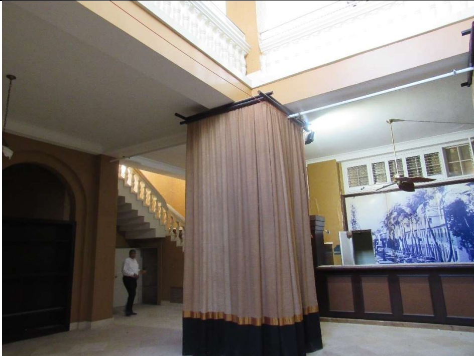
Photo #16 Gulfstream Hotel Building 1 Lake Ave, Lake Worth, FL 33460 Lobby area facing SE (11/7/2019)
