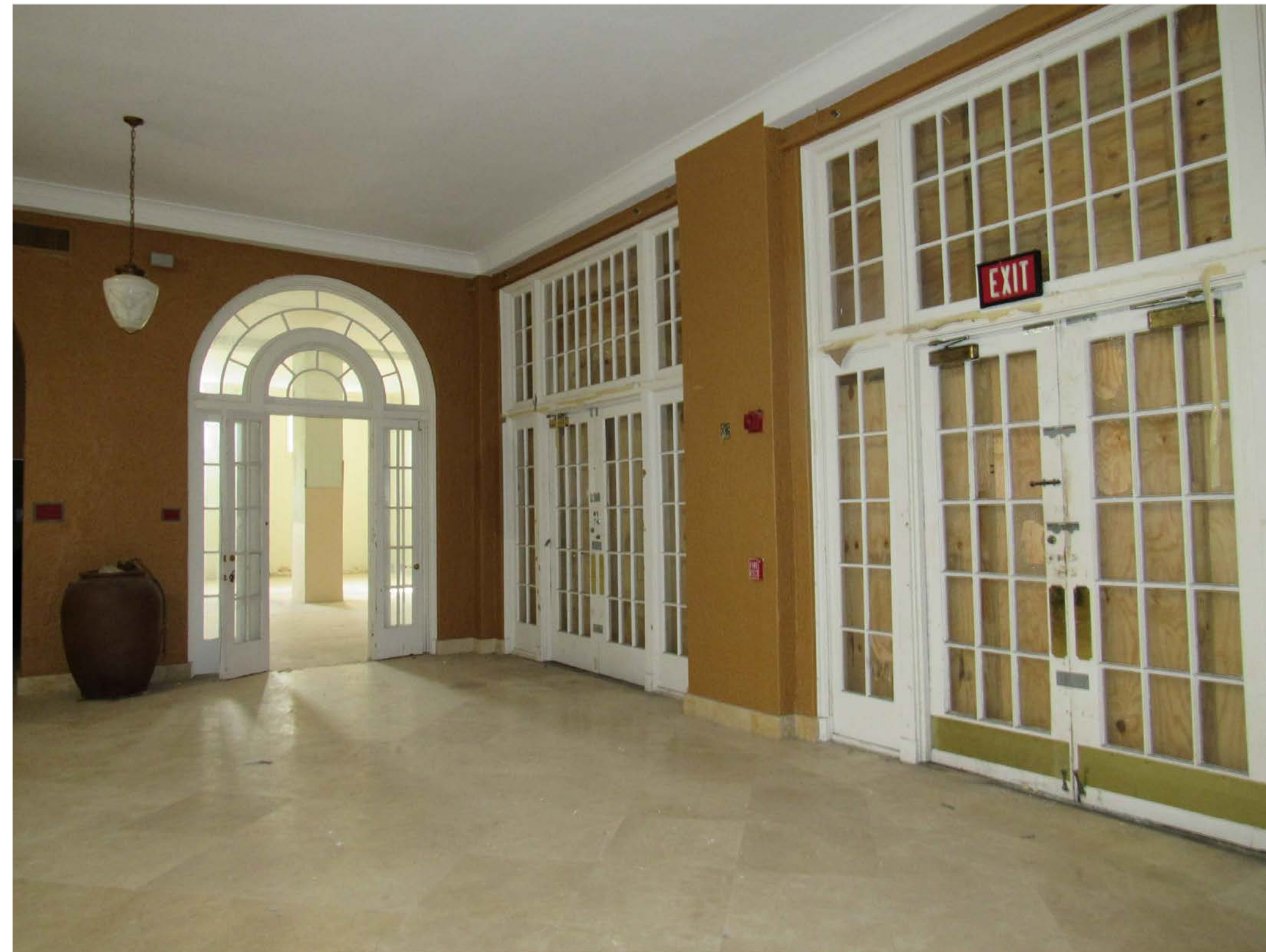
EXISTING FRENCH DOORS TO BE REPLACED WITH NEW DOORS (MULLION CONFIGURATION TO MATCH EXISTING)
