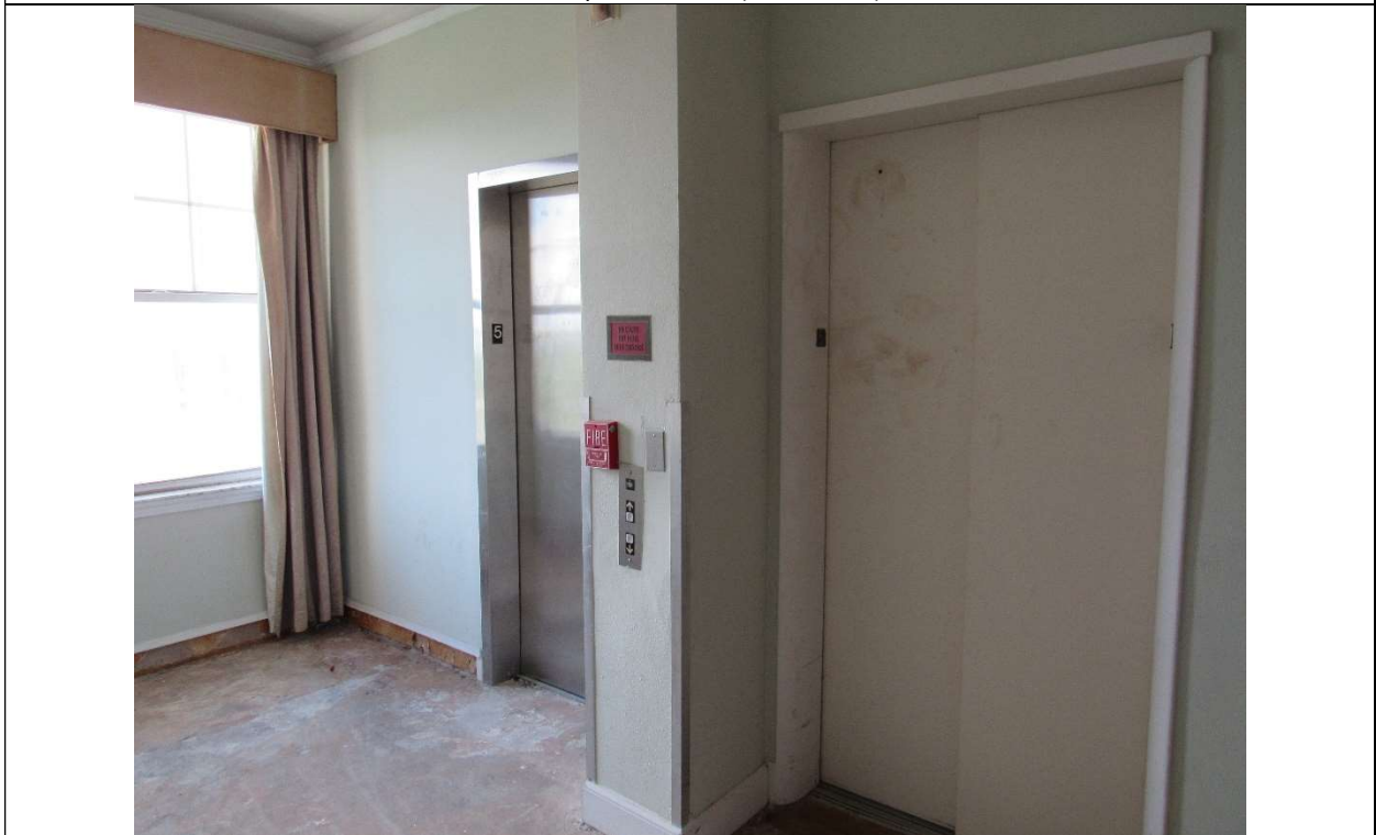
Photo #61 Gulfstream Hotel Building 1 Lake Ave, Lake Worth, FL 33460 Fifth Floor elevator lobby (7/10/2020)
