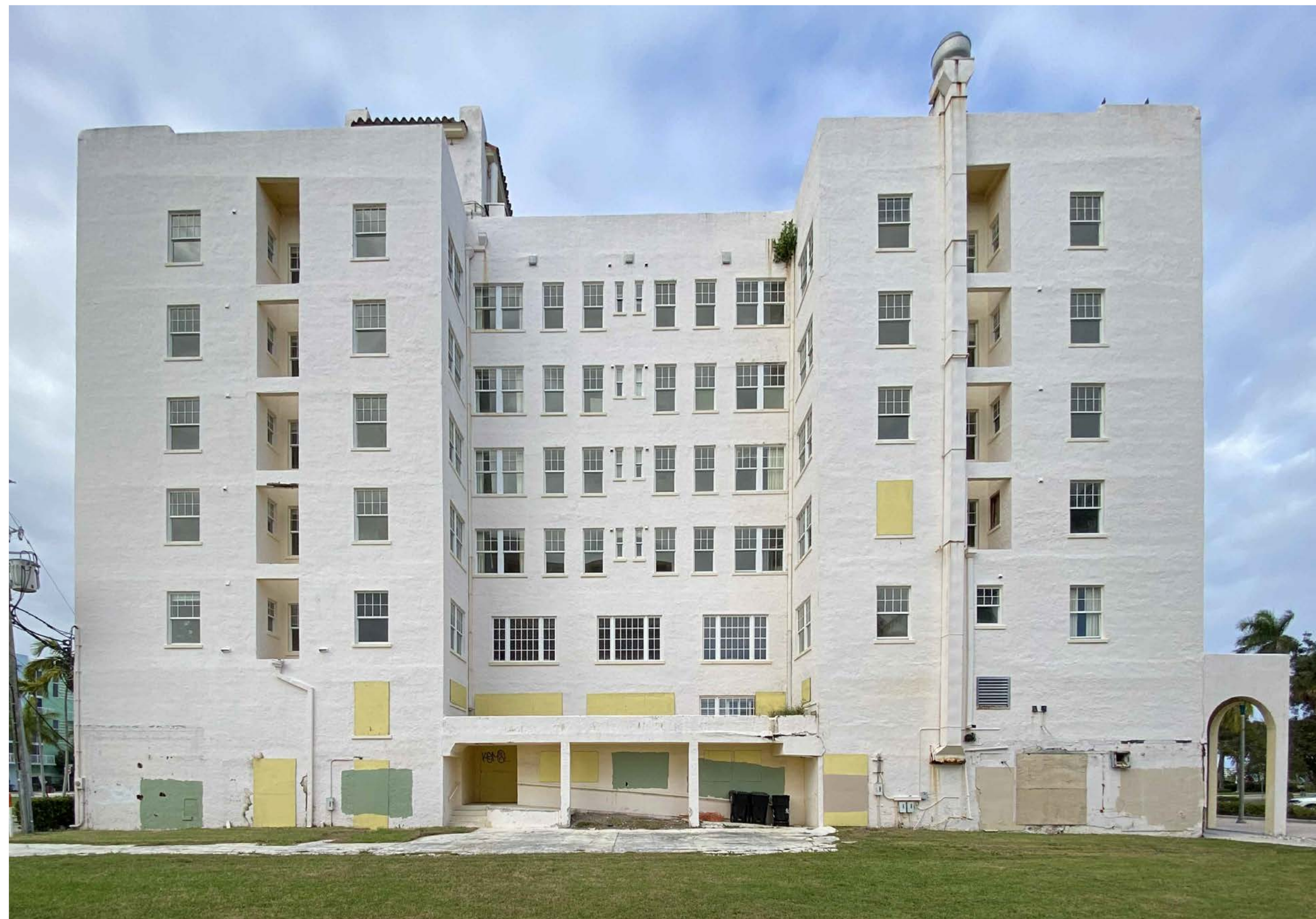
EXISTING BUILDING LOOKING NORTH EXISTING WINDOWS TO BE REPLACED WITH NEW WINDOWS (MULLION CONFIGURATION TO MATCH EXISTING) EXISTING BACK OF HOUSE TO BE RECONFIGURED
