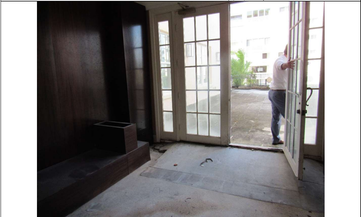
Photo #45 Gulfstream Hotel Building 1 Lake Ave, Lake Worth, FL 33460 Mezzanine level exterior door (7/10/2020)
