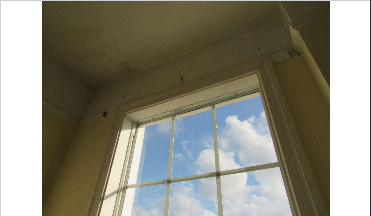
Photo #67 Gulfstream Hotel Building 1 Lake Ave, Lake Worth, FL 33460 Fifth floor window detail (7/10/2020)
