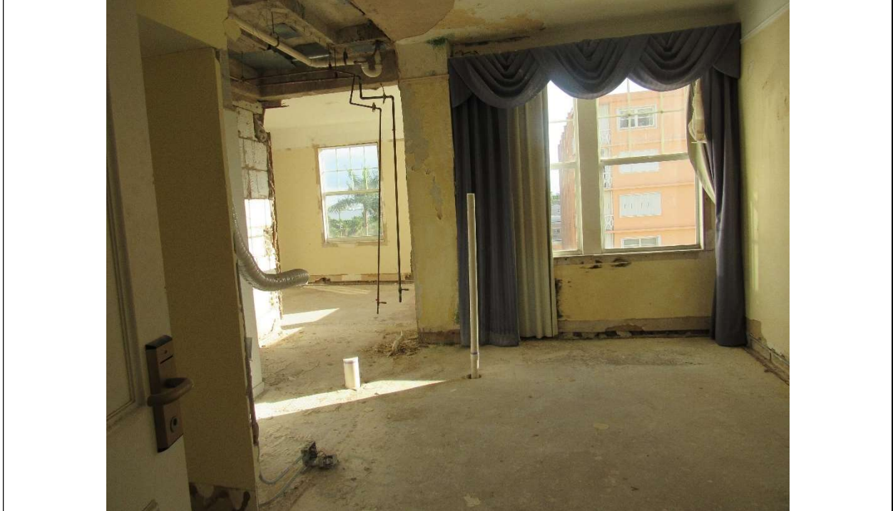
Photo #58 Gulfstream Hotel Building 1 Lake Ave, Lake Worth, FL 33460 Fourth floor room (7/10/2020)
