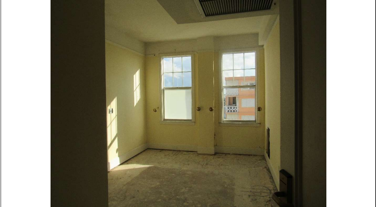
Photo #64 Gulfstream Hotel Building 1 Lake Ave, Lake Worth, FL 33460 Fifth floor room (7/10/2020)
